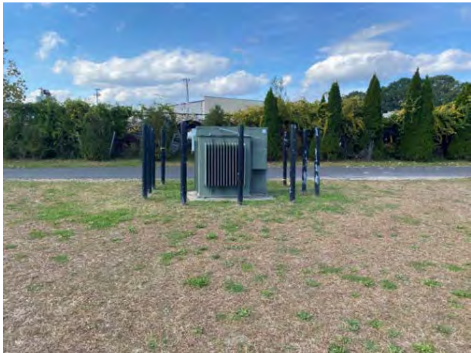
Example pad-mounted transformer along the western portion of the Site.
