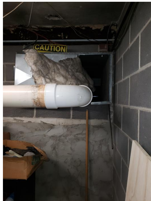
PVC Vent Into Duct
